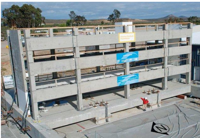
Fig. 10 Three story was erected by precast concrete structure. Reproduced with the permission from [113].
