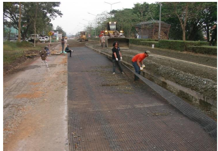
Fig. 1 Asphalt Road reinforced using Miragrid GX100/100 geogrid (Photo from the field construction by the authors [8] ).
